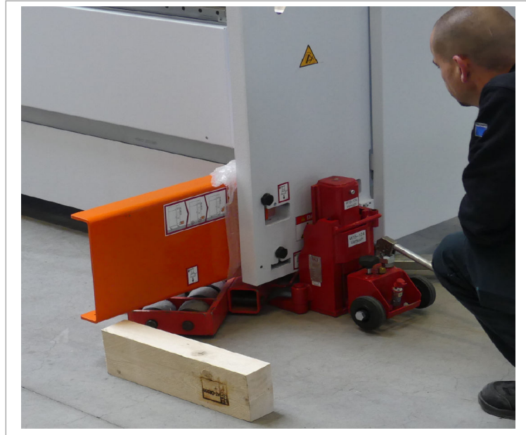
Position of the hydraulic hoisting jack
